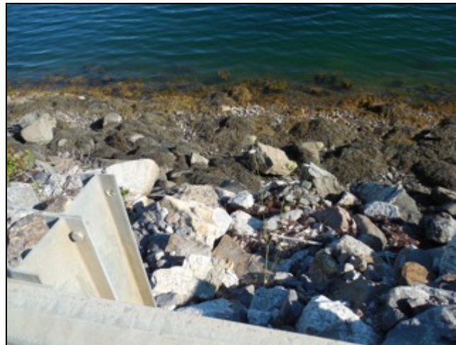
Rocks recently tumbling away from dam face are obvious due to lack of seaweed growth - July 2015
