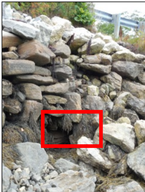
Sloughing off seaward face reveals original cribbing - July 2015
