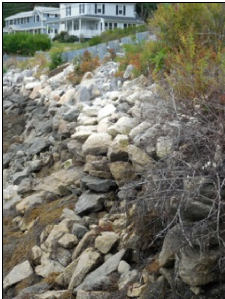
Outward movement of rock visible all along seaward face of dam - July 2015
