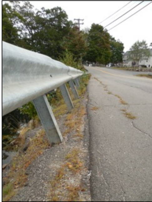
Slumping dam structure cracks pavement and splays guard rail stanchions (July 2015)
