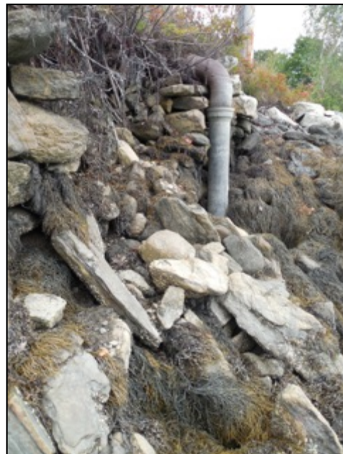
Bottom of seaward siphon now fully obscured by fallen rock - July 2015
