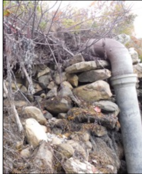
Outward moving rocks wedged against seaward siphon - July 2015
