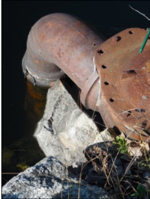
Outward moving rock wedged against lakeside siphon - July 2015
