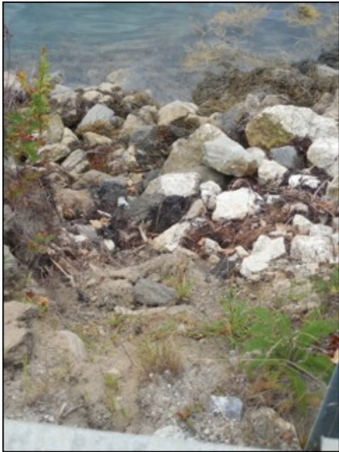
Rock falling away from dam face narrows the roadbed (July 2015)
