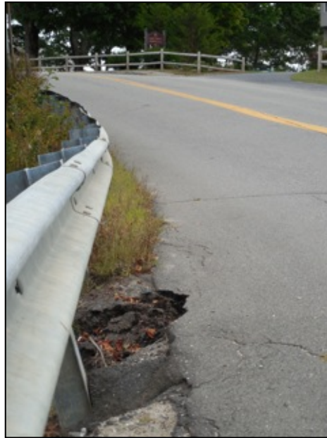
Erosion along narrowed road bed encroaches under the guard rail to the pavement on the lake side (July 2015)
