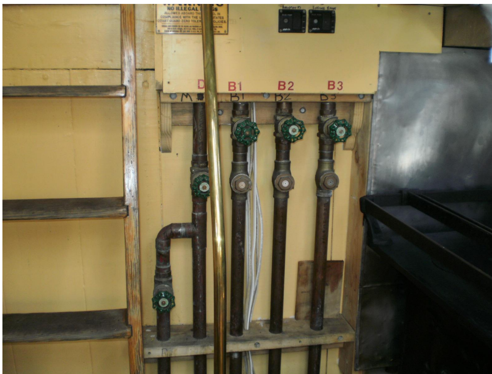
VIEW OF NEW MANIFOLD SYSTEM IN THE ENIGNE ROOM
